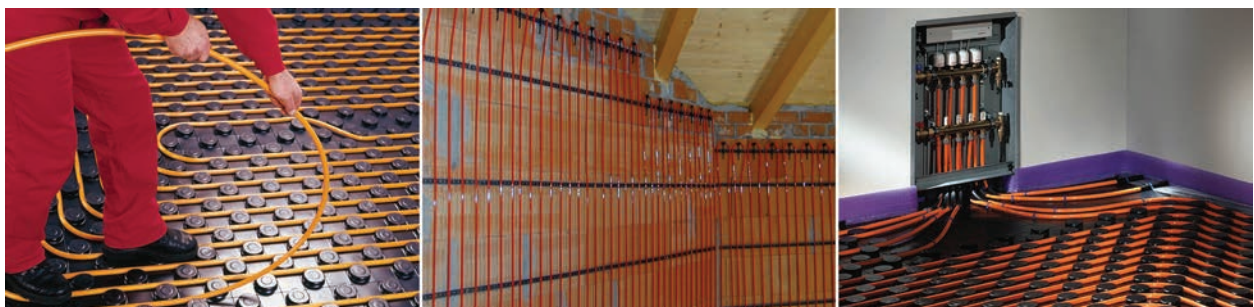
Heating and Cooling
