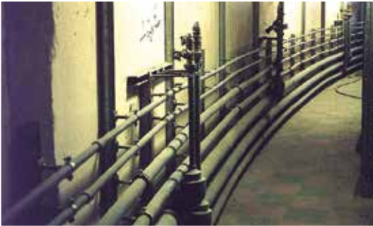
PB-1 was selected because of its flexibility, allowing to smoothly follow the unique shape of the building.
